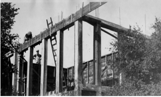
La Casa Roca under construction showing reinforced concrete framing, arroyo stone walls and timber joists.
